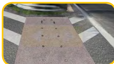
Base in cemento prefabbricata
