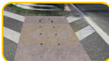
Base in cemento prefabbricata
