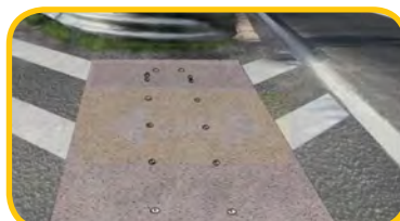
Base in cemento prefabbricata
